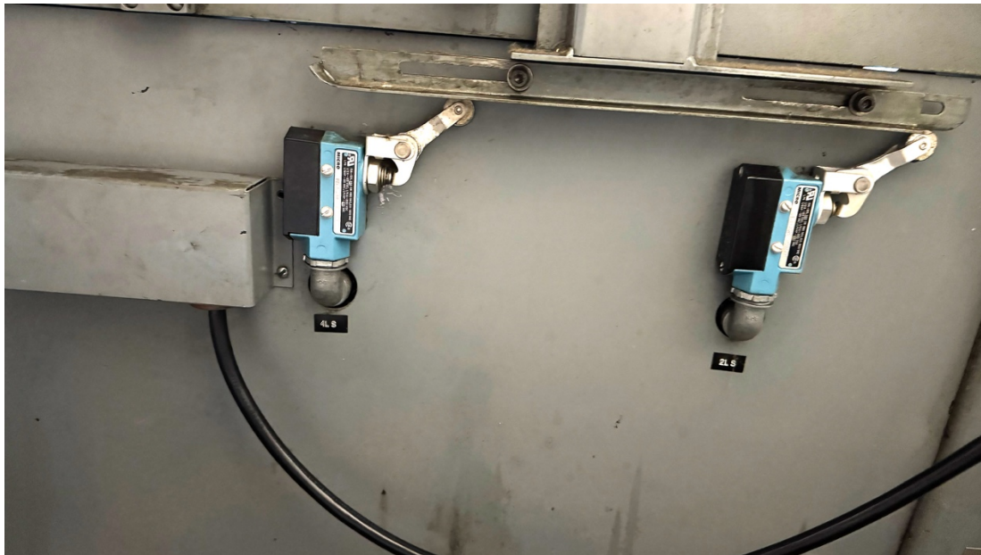
Figure 30: The micro-switches on the back of our press at the feed board end. These are switches 4LS - Rev. Slow (left) and 2LS - Rev. Stop (right) in the schematic. 4LS informs the control circuit that the carriage is approaching the feed board, and 2LS informs the control circuit that the carriage is all the way back to the feed board. These are replacement microswitches from those originally installed on the press and are shown in the position where they are both engaged (pressed) by the cams on the carriage. You can adjust where the carriage engages these switches by moving the cams back and forth.
