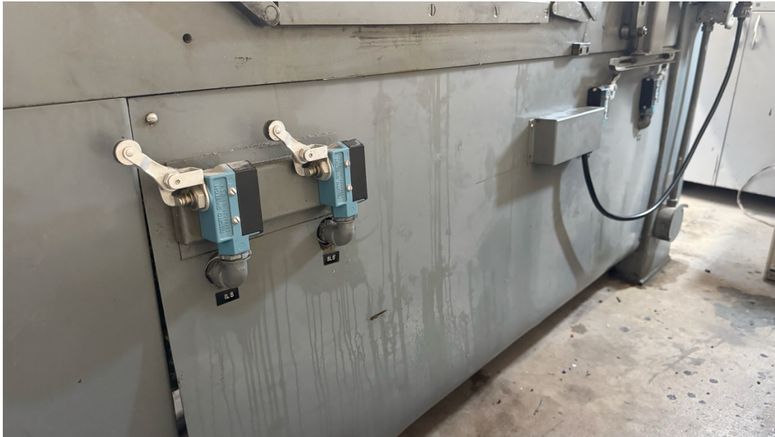
Figure 31: View of the back of our Vandercook Universal I showing (replaced) microswitches 1LS – For. Stop (left), indicating that the carriage is all the way to the end of the press bed), and 3LS – For. Slow (right) indicating that the carriage is almost to the end of the press bed when moving forward.
