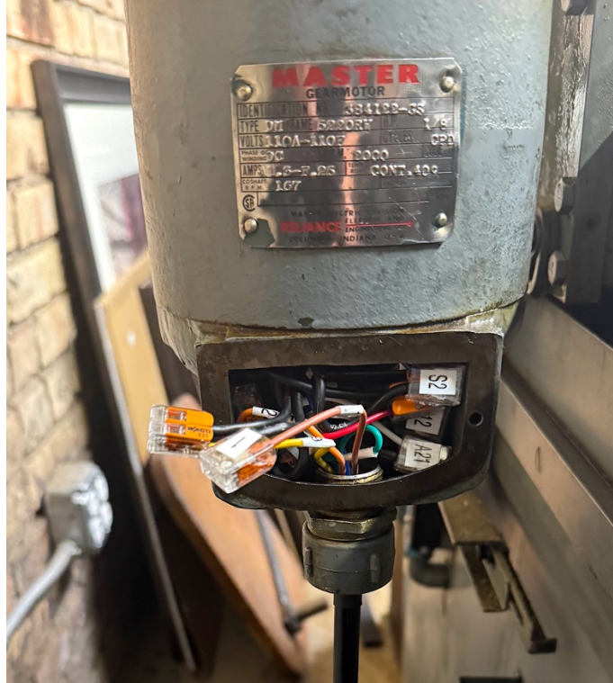
Figure 55: This shows the cable wires connected to the drive motor using Wago lever splices. These are very handy and very solid connections and are easily removable if, for any reason, you want to change things. I stuffed them all in the motor wiring cavity and replaced the plate on the outside.
