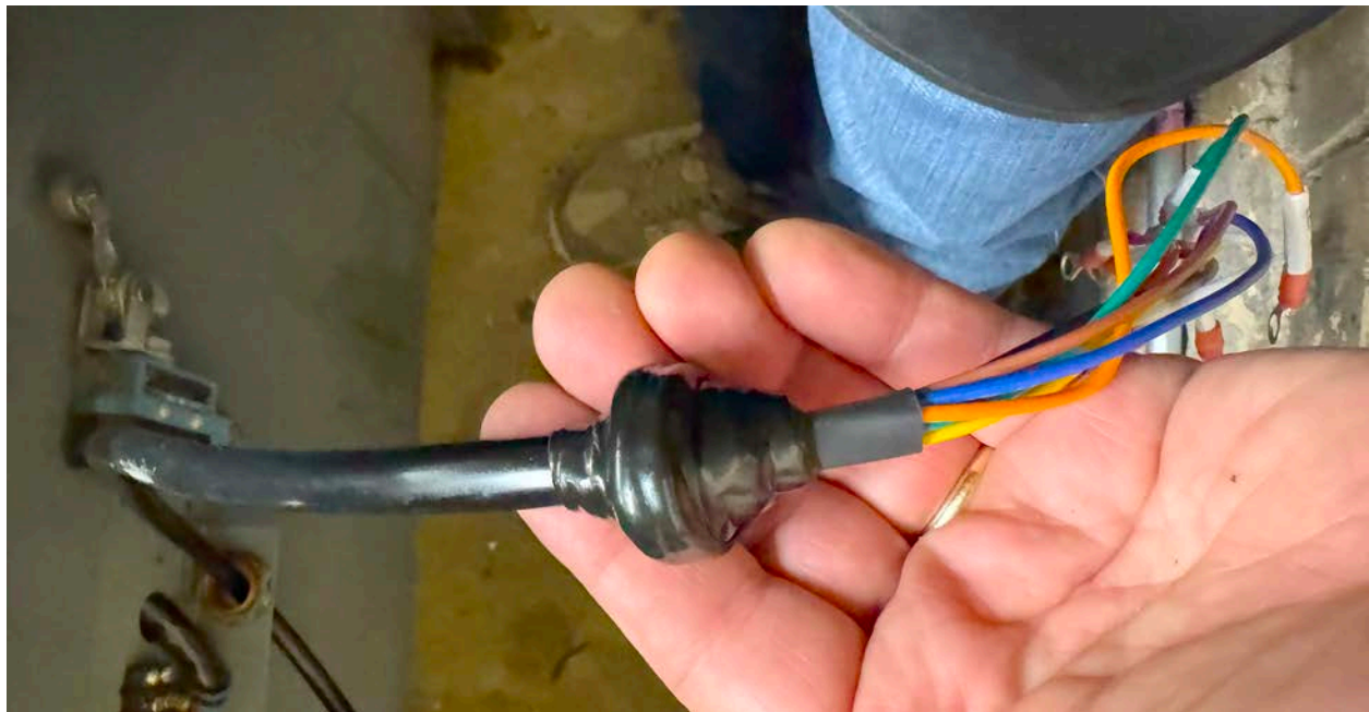
Figure 56: This shows the thickening ring on the press-end of the cable. I used a cardboard ring which I then wrapped with rubber self-fusing tape. This ring sits on the mounting flange and lets the cable rotate freely as the press carriage moves back and forth, but does not allow the cable to pull directly on the screw connections to the barrier block.
